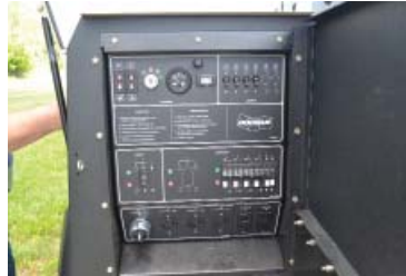
Protected control panel
