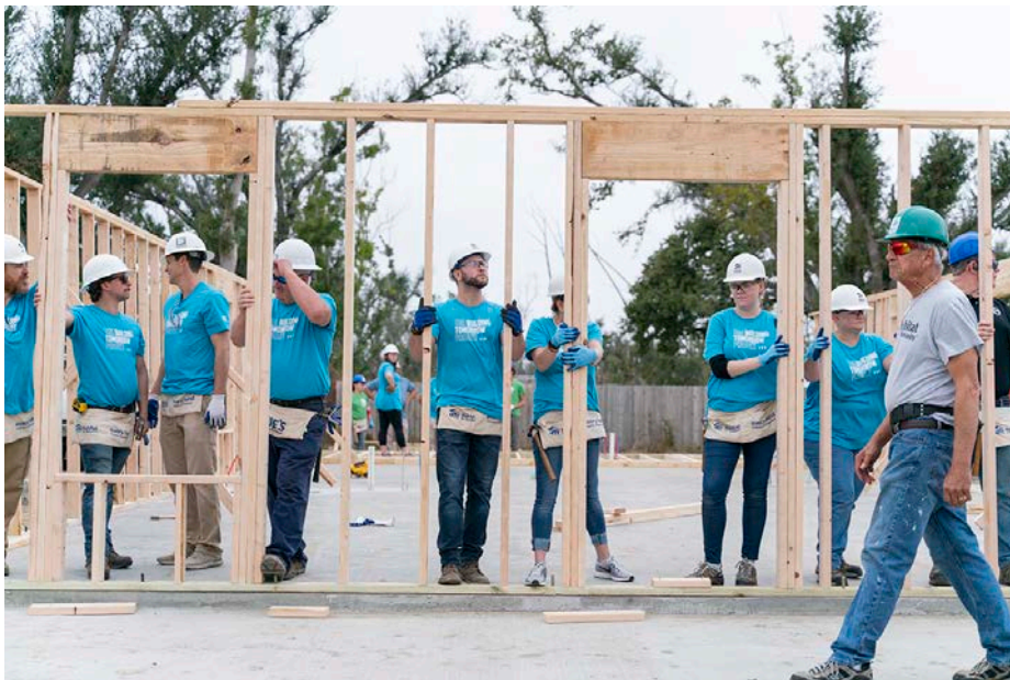
Cowin Equipment volunteers raise and secure the external wall on the front of Emma Andreazzi's new home in Panama City.
