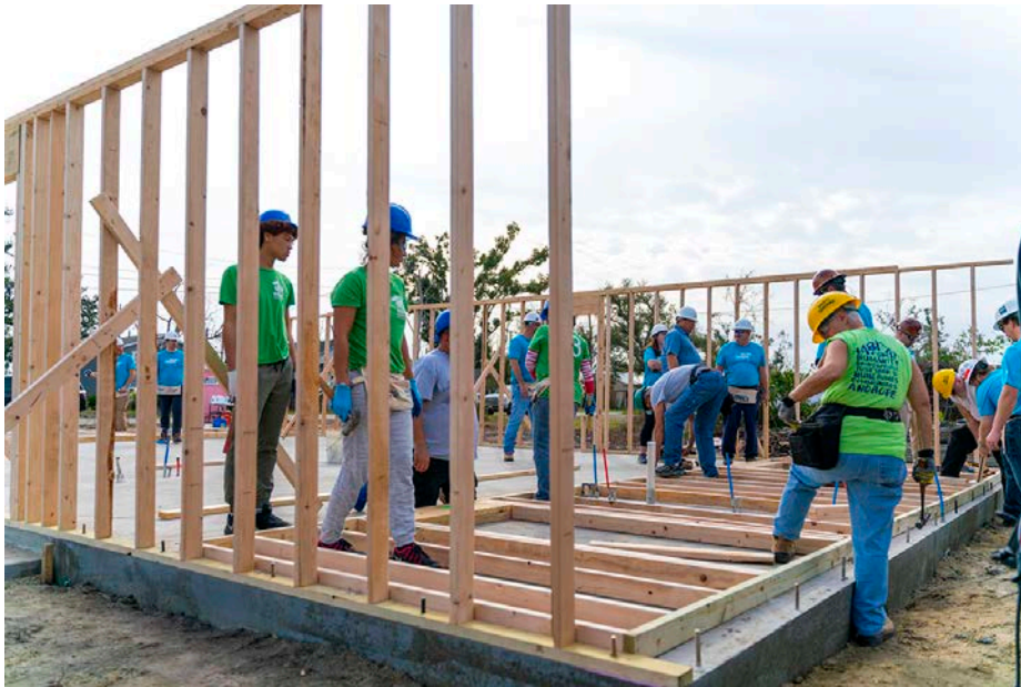
Cowin Equipment volunteers finish one of the external walls on a home for Emma Andreazzi of Panama City.
