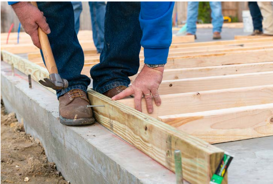
Cowin Equipment volunteers worked to frame in and raise the four external walls on one of the Panama City builds.
